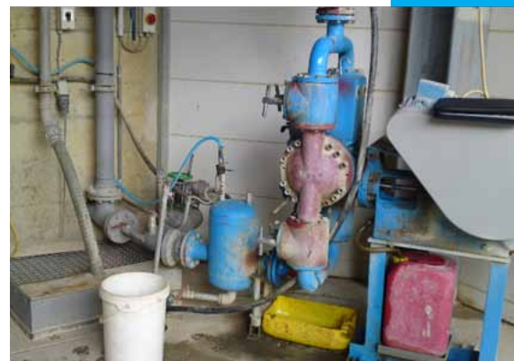
the replaced Abel pump
